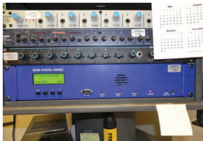
At work in the rack.
